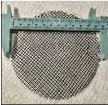
One of three wire screens in the air ducts of the heater system.
