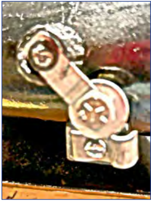
Cable attachment clamp on the heater box inlet damper. Cable is not shown.
